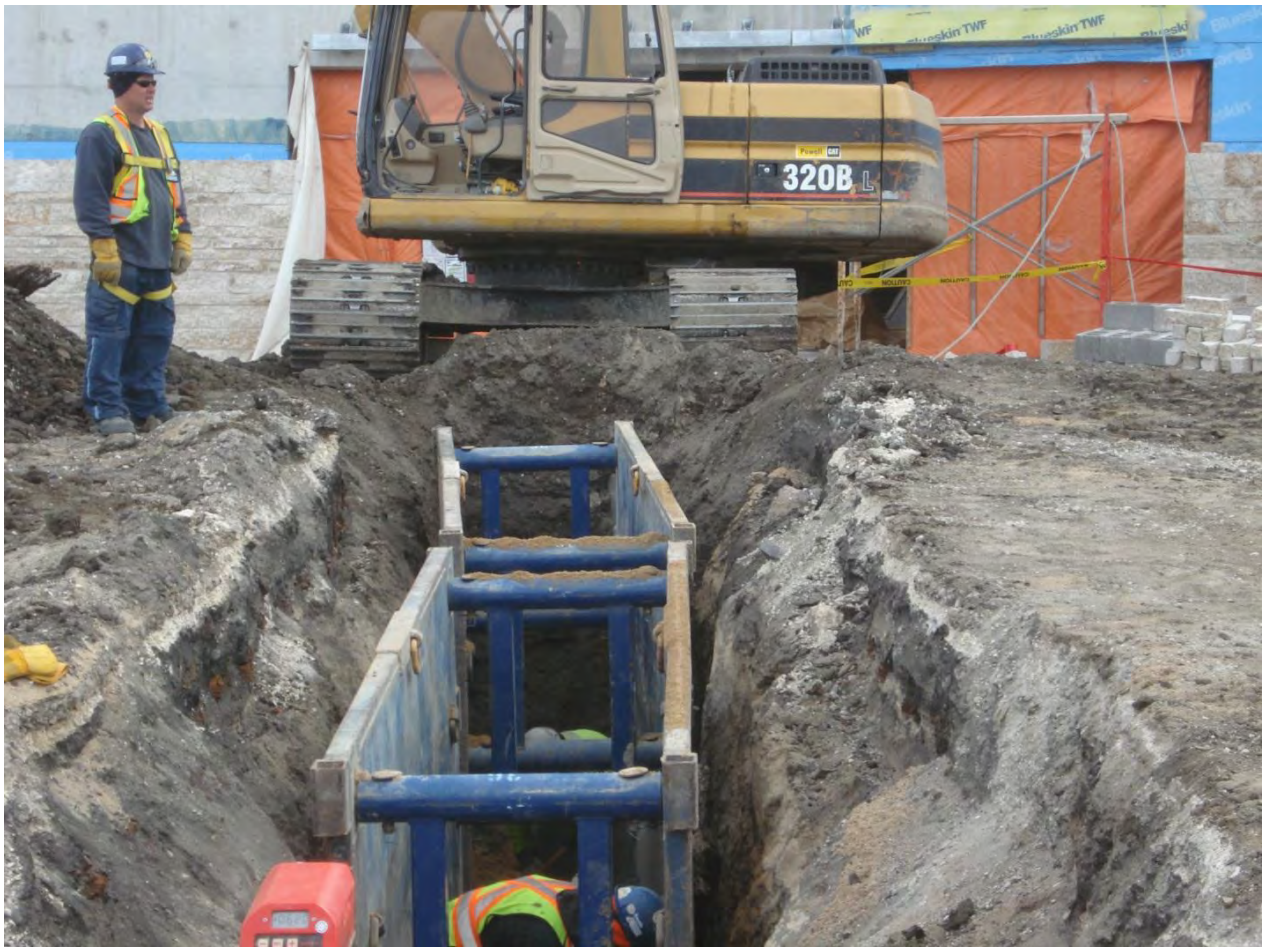
Photo 15-17: Installation of land drainage system from Manhole 6 to Catch basin 1 on the north side of Root A.
